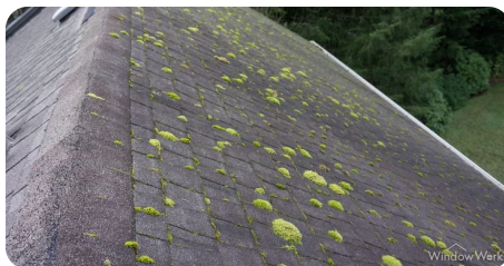
Green clumps: moss. The number one roof problem here. It anchors into the granule layer and lifts it as it swells and dries.
