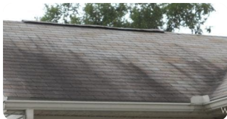
Black streaks: algae. Feeds on the mineral filler in the shingle. Mostly cosmetic at first, but it holds moisture and it spreads.
