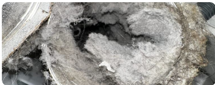
A duct packed end to end. The dryer was still running, just working far harder than it should.
