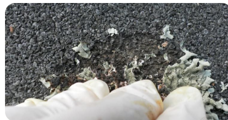
Crusty gray patches: lichen. Bonded down into the shingle. Scraping it takes the protective granules with it, as here.
